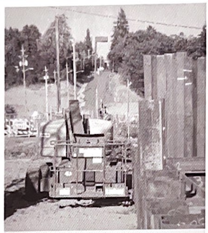
With the 39 th St hill in view behind the cherry picker, progress is evident on the overpass project, which should be completed by the winter of 2010.
