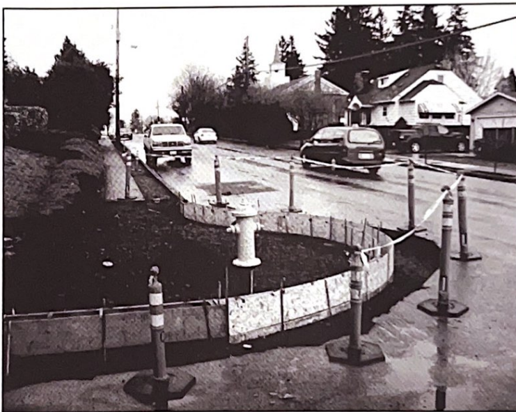
Rainy days won't slow the pace of construction along 39th Street, where a total of $620,000 in state and local funding will make the highly travelled roadway safer for vehicles, pedestrians and bicyclists alike.
